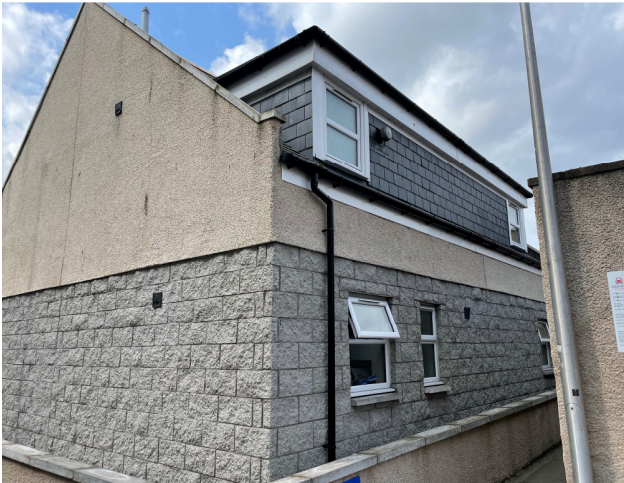
a) Two storey building immediately to the South East, 9-11 Charles Street. Modern dry-dash render & fystone.
